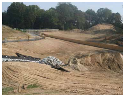
Poorly managed construction sites allow sediment to run off into nearby waters.
