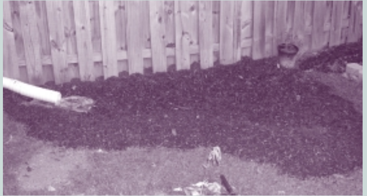
Same rain garden immediately after excavation and soil amendments and mulch added, prior to planting
