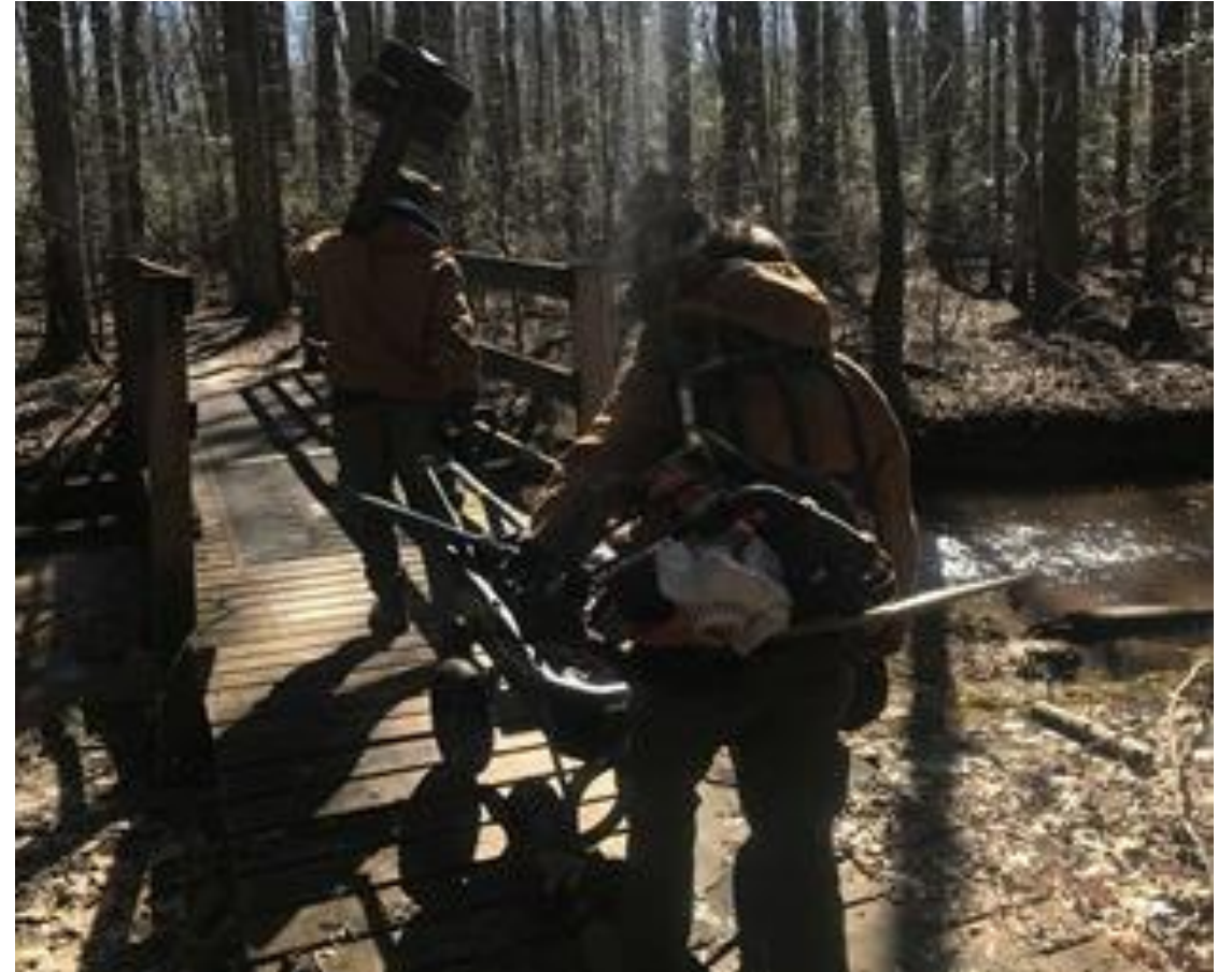
Project Specialist Gray and Kozak carrying Wayfinding sign and drill auger in a remote part of Cedarville State Forest. Many of the Wayfinding signs required hand transport of materials and equipment in many parts of Maryland State Parks as vehicle access is difficult.
