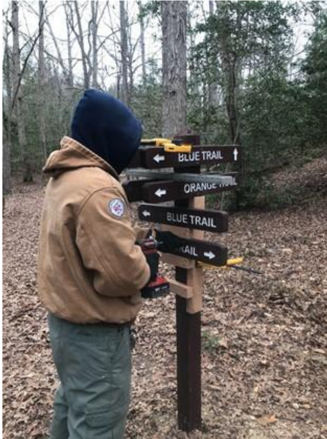
Project Specialist Gray using a level and jig the MVCC developed to ensure Wayfinding signs remain in accordance with Maryland Park Service standards.
