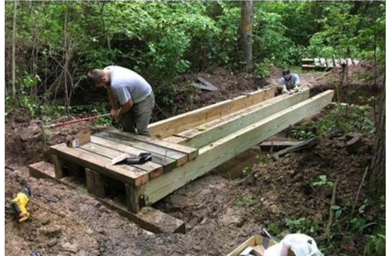
Project Lead Ulery and Project Specialist Gray constructing a 20-foot long, 6-foot wide, equestrian rated wooden bridge at St. Mary's River State Park.
