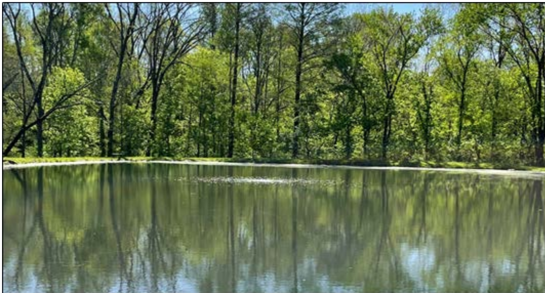
Brunswick Pond aerator in operation
