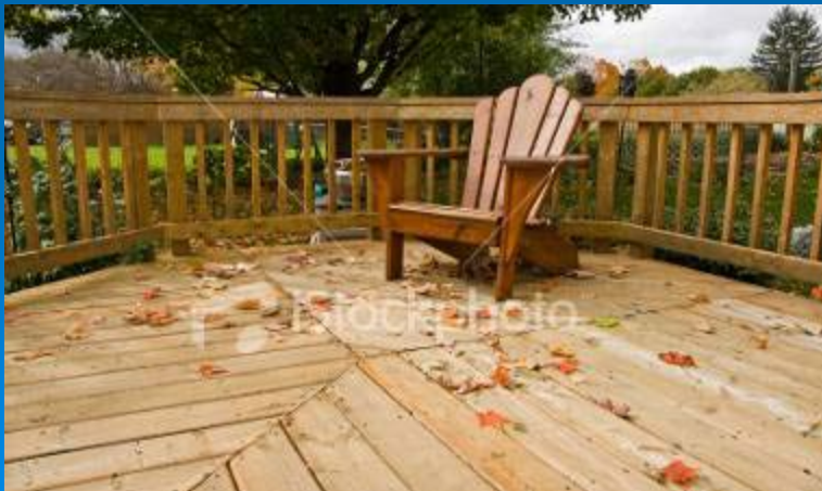
DECK WITH GAPS
