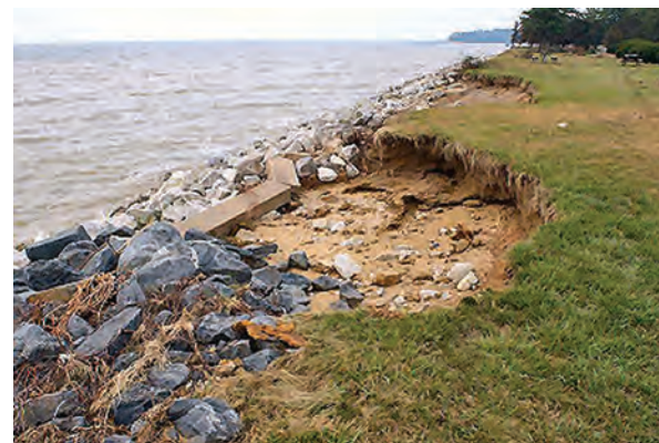
Shoreline erosion from storms.
