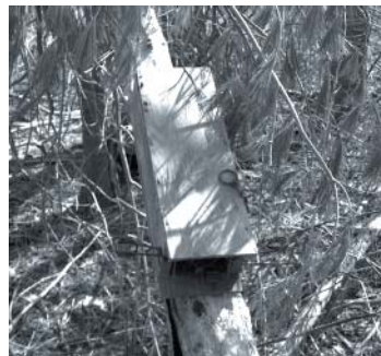
Leaning pole set
