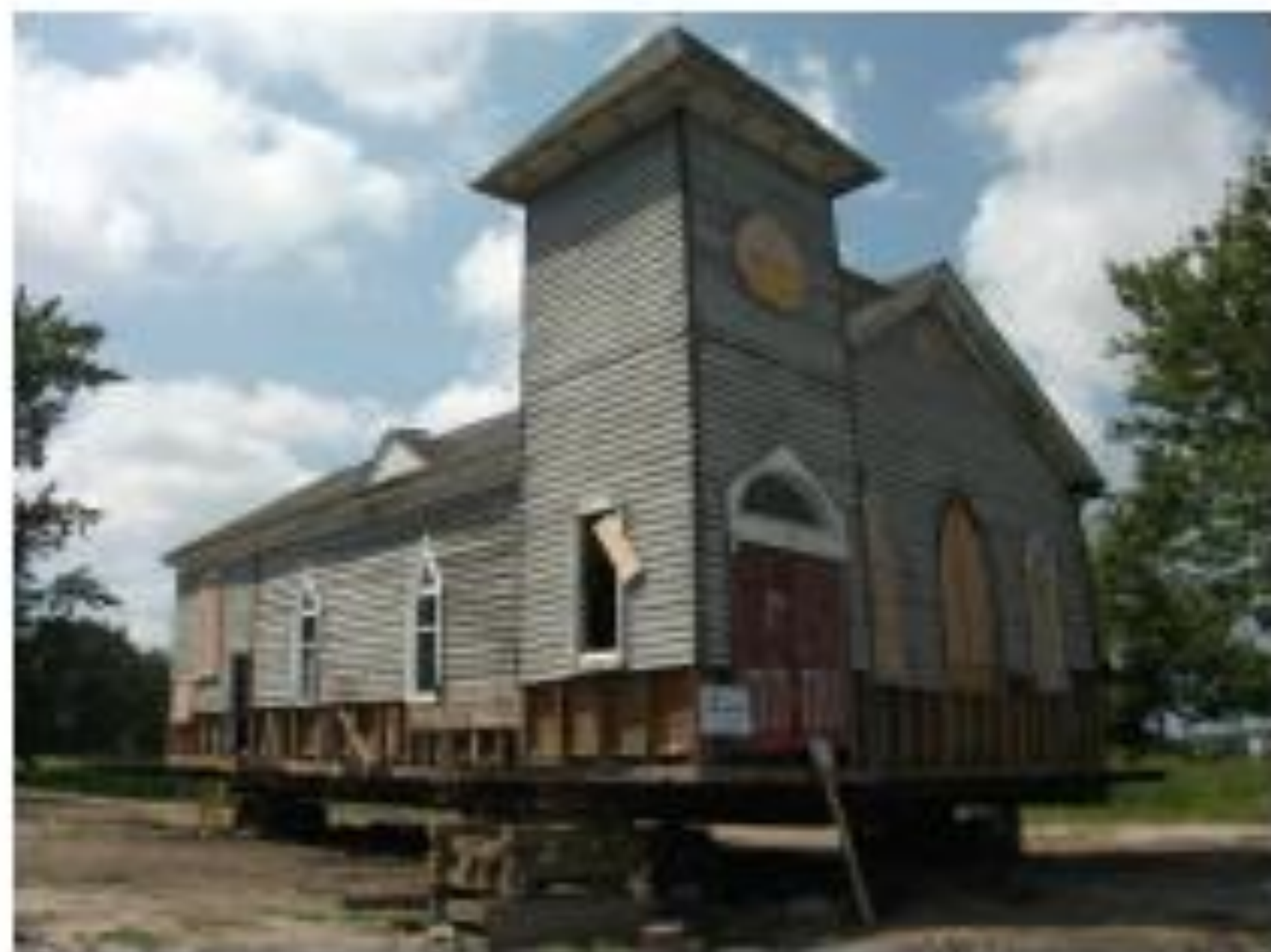
Above: Church during lifting and foundation repairs phase in the fall of 2012.
