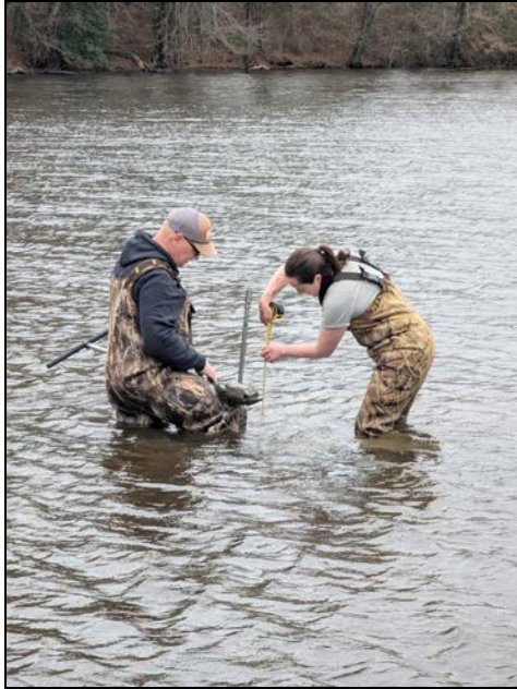
Eastern Regional staff working on deepening the pond at Cypress Branch Natural Resources Management Area.
