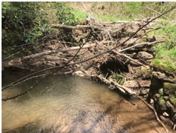
Collapsed culvert on the South Branch Bear Creek and downstream bank scour caused by the blockage during high flow events.
