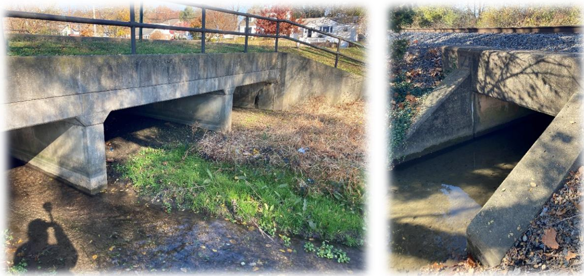
Figure 4: Culvert Leaving Northern Middle School (left) and Culvert under Railroad East of Maintenance Yard (right)
