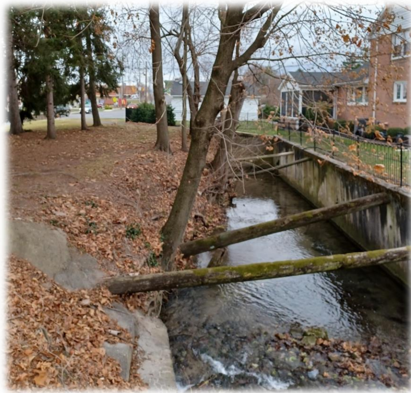
Figure 5: Failing Retaining Wall Supported by Telephone Poles
