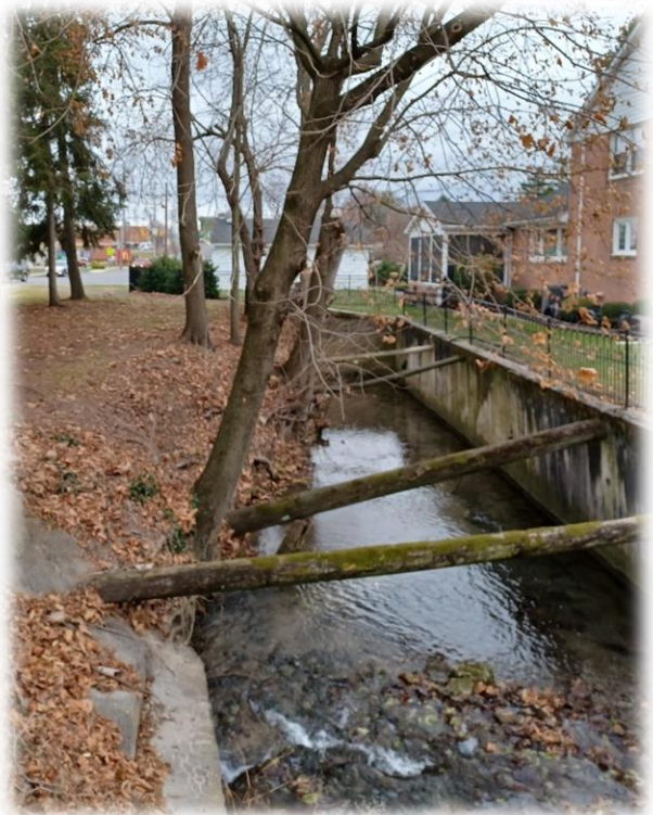
Figure 15: Failing Retaining Wall
