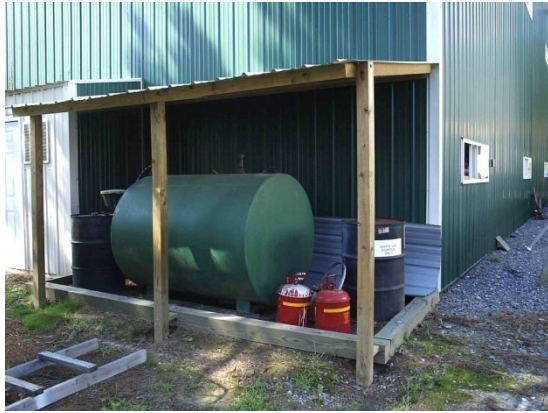
Neat, clean liquid recycling tanks.
