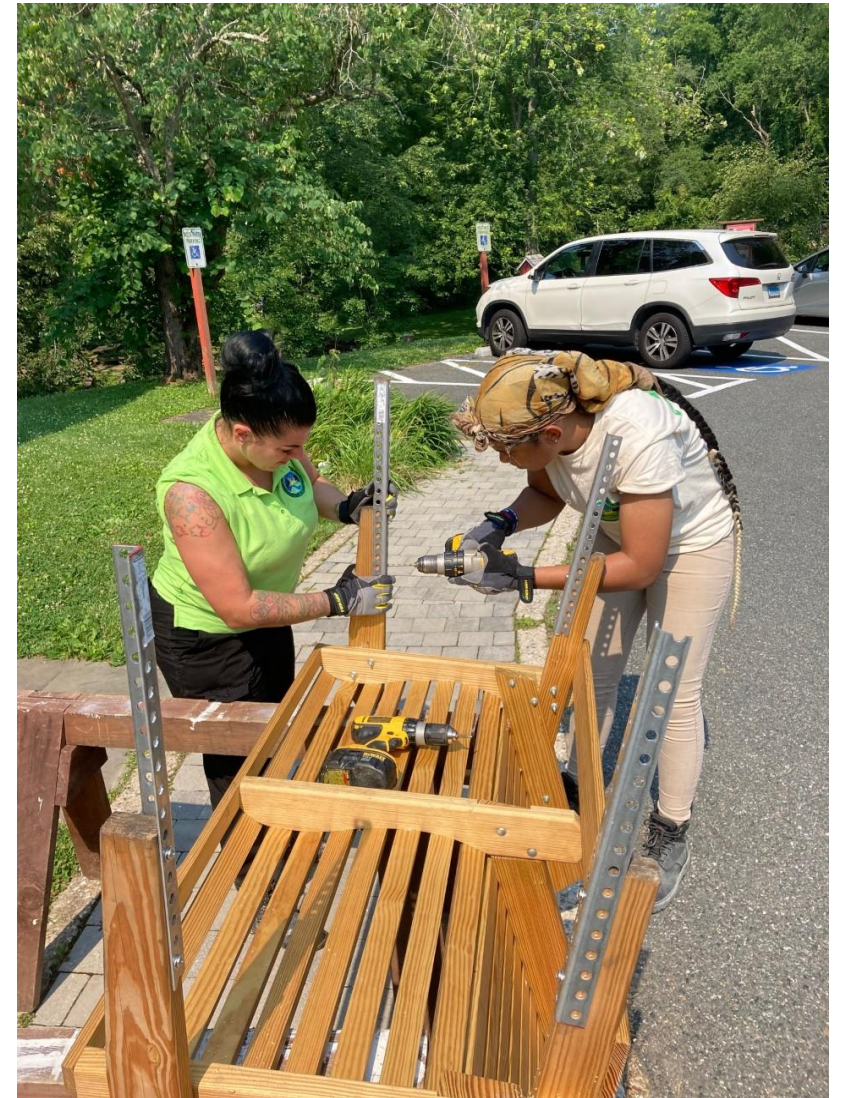
Gunpowder Falls Crew Member and Leader work together to prepare a bench for installation.
