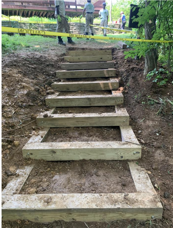
Step 4: Steps are installed, time to fill with stone dust and tamp.
