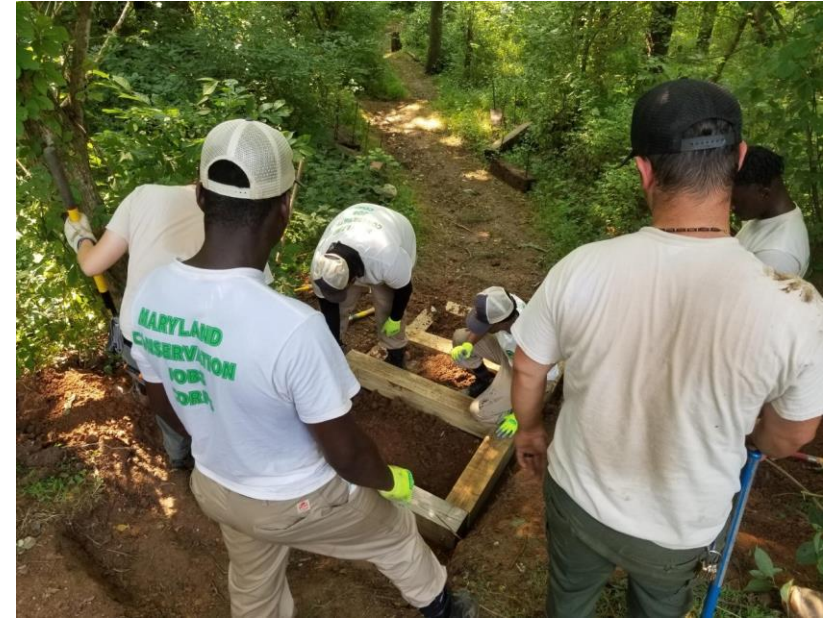
Step 3: Level, install, and fill new steps with a little help from your friends.
