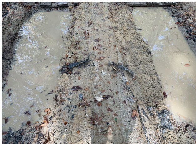
Example of road conditions after rain.
